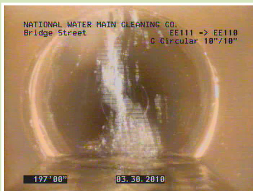
Infiltration Gushing through Pipe Joint
