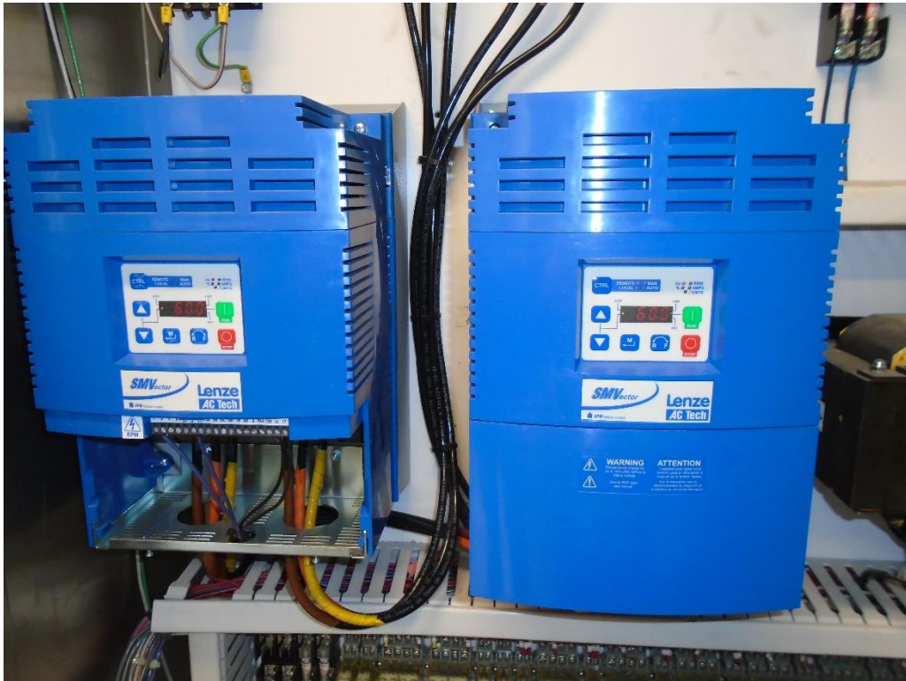
Variable Frequency Drives (VFD's)
