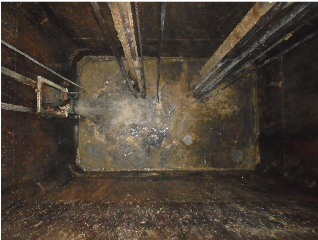
Wet Well (Inside)
