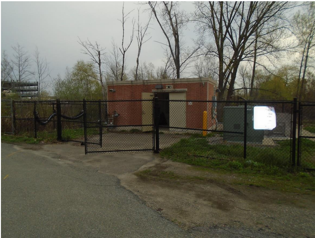
Rustcraft Road Pump Station Exterior (Front)
