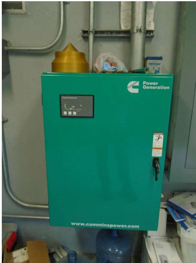
Automatic Transfer Switch
