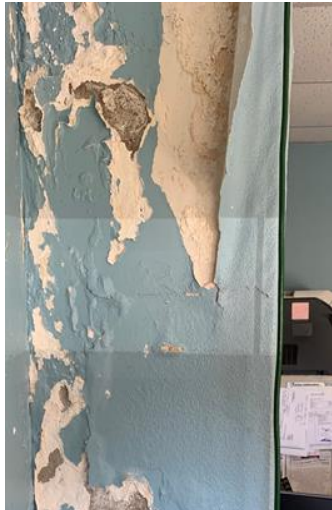
FIRE: Perpetual water damage from the tower
