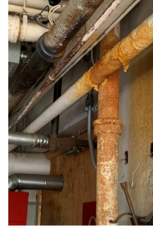
BOTH: Deteriorating ceilings, walls & pipes.
