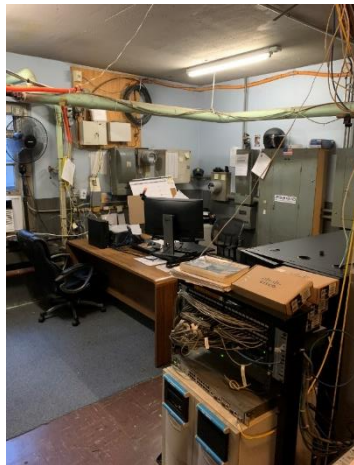
BOTH: There are offices located in the electrical room and critical IT equipment in spaces with no HVAC.
