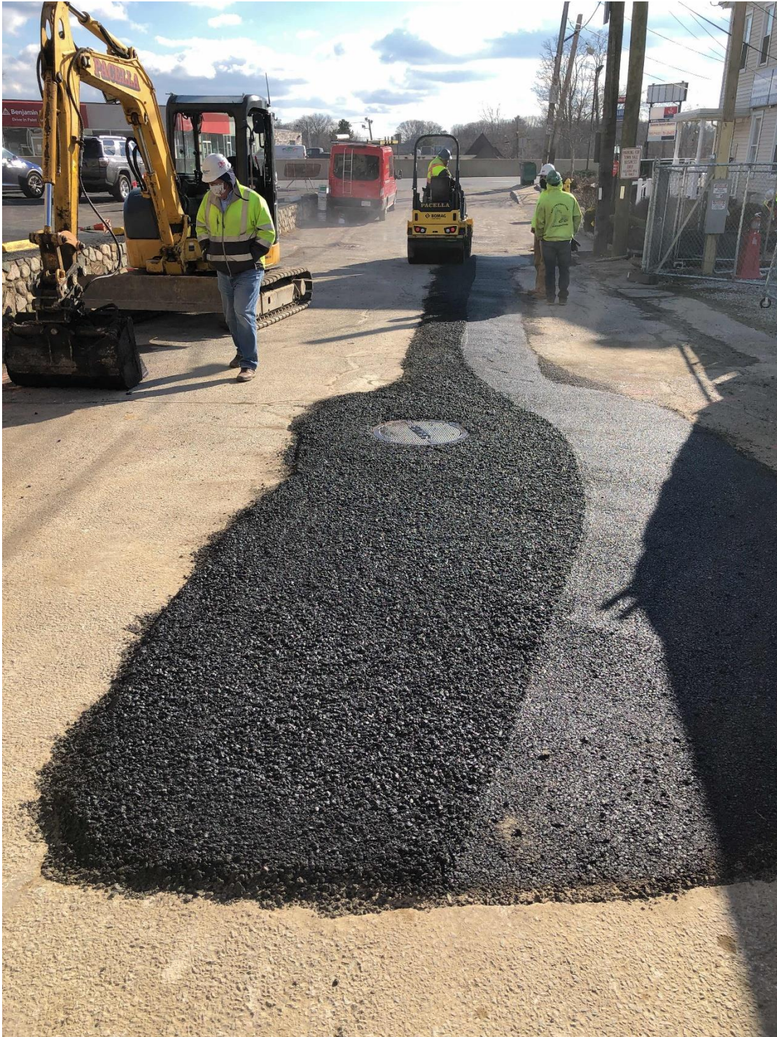
DPW crews re-routed existing to remain sewer line at 1 Union Place to off-site.
