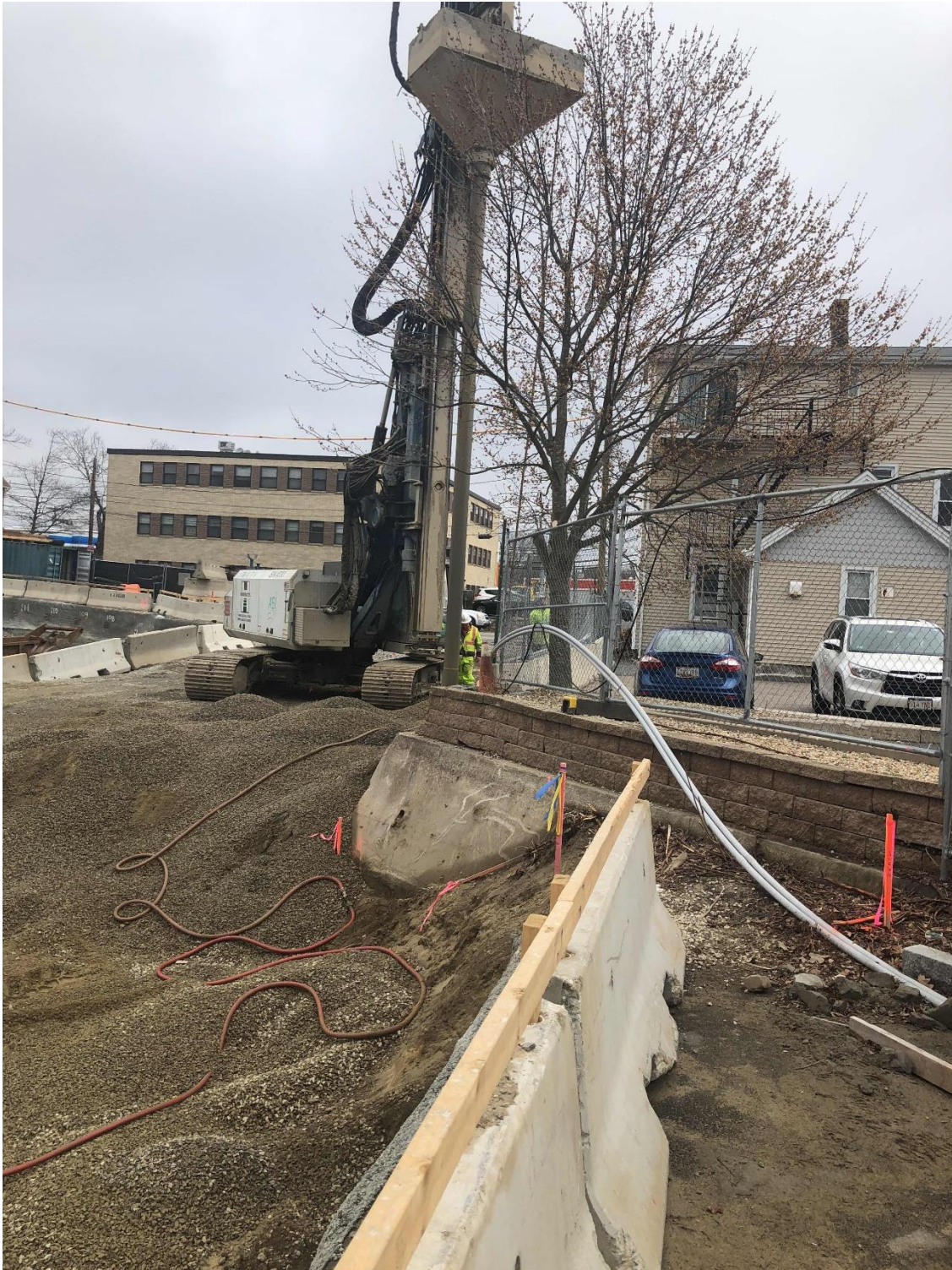
RAP install along 1 Union Way property line. Abutter's retaining wall footing over the property line.
