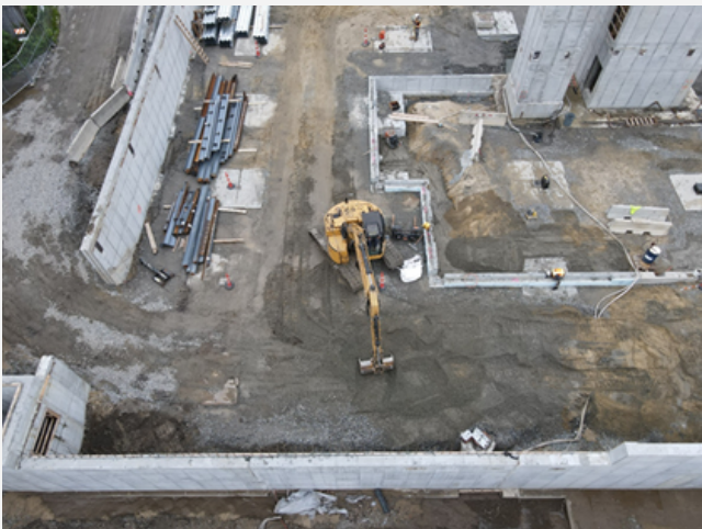
Caption: Aerial photo of construction site taken on July 13, 2021. Activities onsite include overall site consolidation, clean-up and preparation for steel installation as shown by the excavator in this photo.
