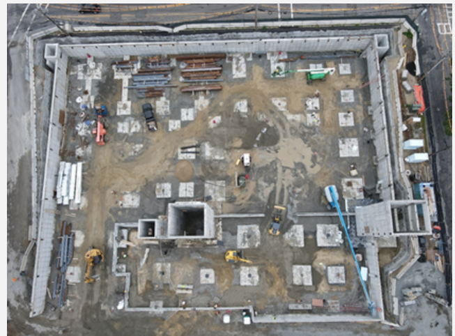
Caption: Aerial photo of construction site taken directly above on July 13, 2021. Pieces of steel are being delivered to the site and securely stored along the west and south walls, shown at the top and left of this photo.
