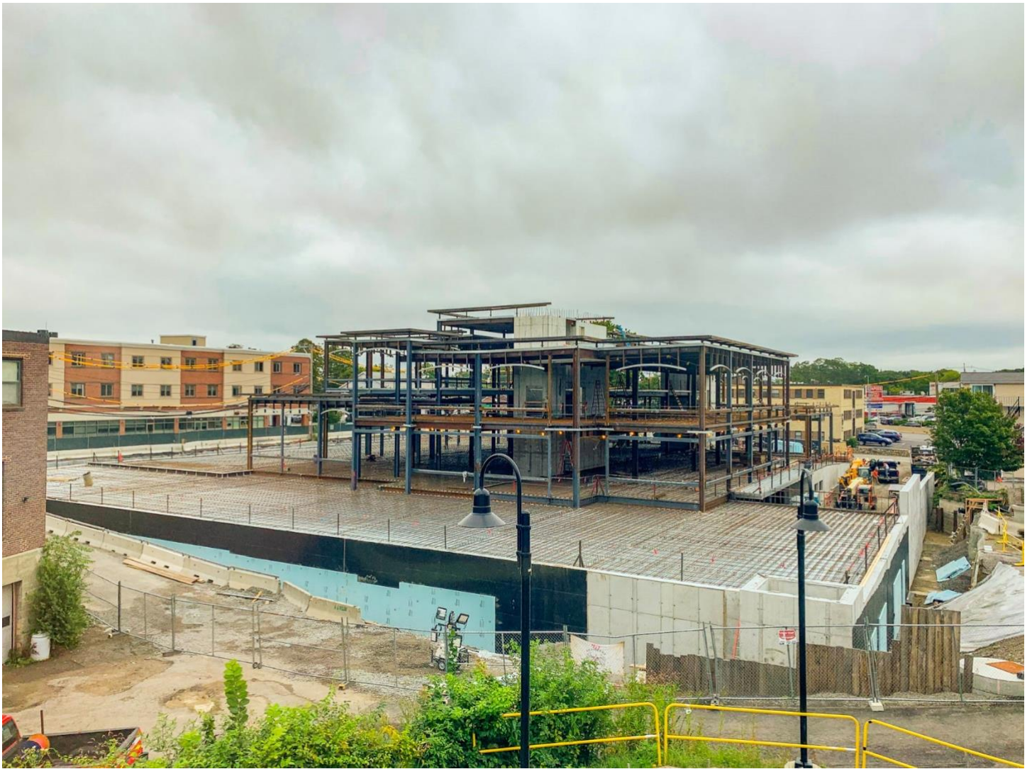
Caption: Photo of active construction site taken from the north side of Town Hall on Friday, September 17, 2021.
