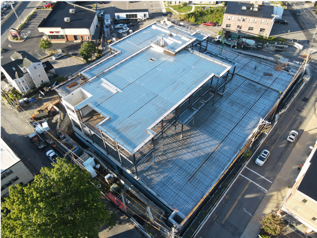
Photo of construction site taken via drone on Monday, September 20, 2021 at 7:45 a.m.
