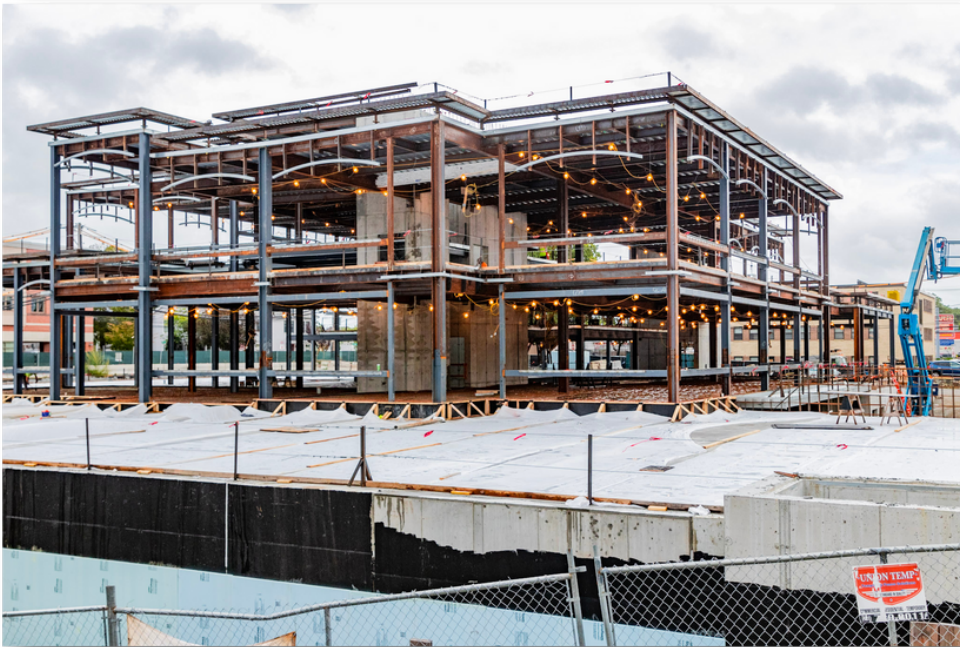
Caption: Photo of active construction site taken from the north side of Town Hall on Friday, September 24, 2021. The signed beam in still visible near the elevator shaft and stairwell at the center of the photo.
