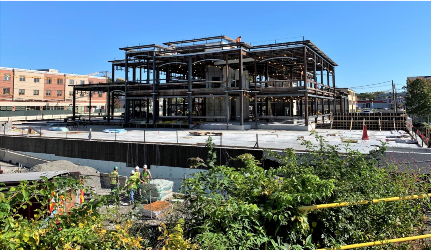
Caption: Photo of active construction site taken from the north side of Town Hall on Thursday, October 7, 2021.
