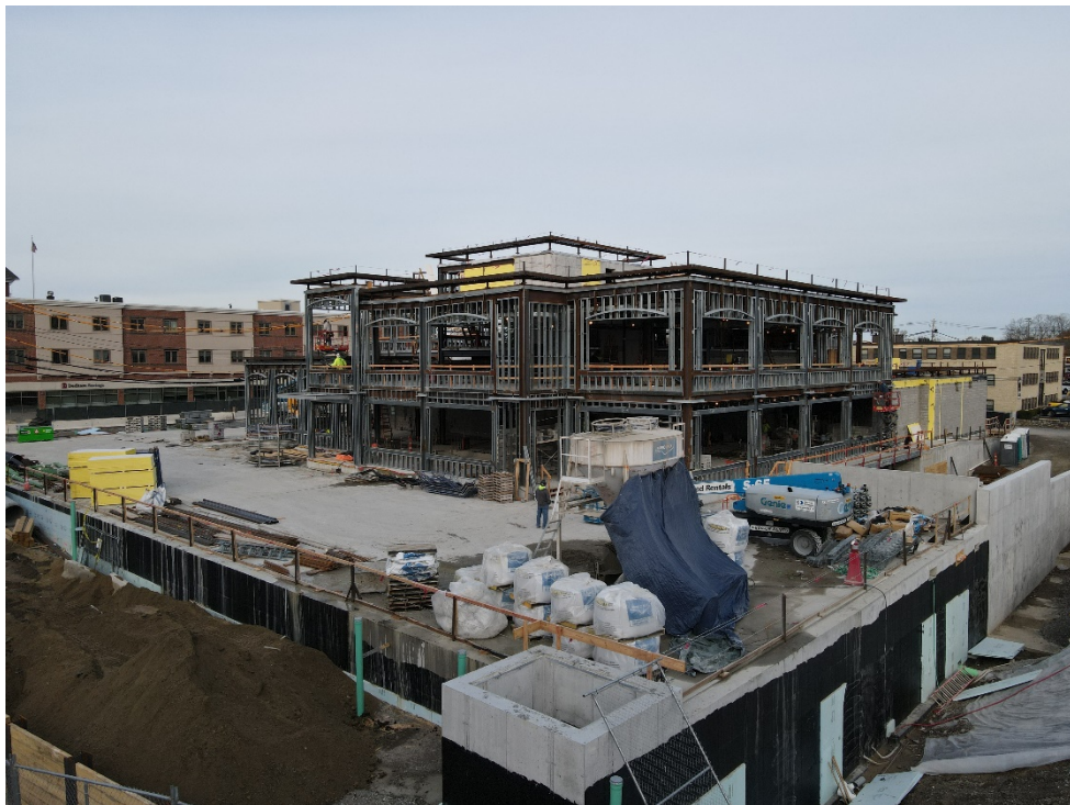
Caption: Photo of the southeast corner of the building taken by drone on Wednesday, November 17, 2021 of the active construction site.
