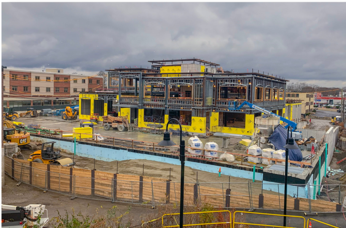
Caption: Photo of the active construction site from the north side of Town Hall on Friday, November 26, 2021. The yellow sections along the exterior walls of the building are the DensGlass sheathing, designed to resist mold and moisture.
