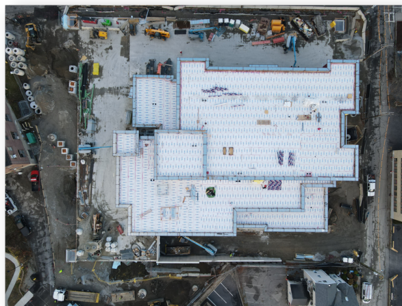
Aerial photo of the active construction site taken using a drone on Friday, December 3, 2021. The white material shown on the roof of the building is the air vapor barrier. As of Friday, December 3, crews had successfully completed the installation of air vapor barriers on the roof.
