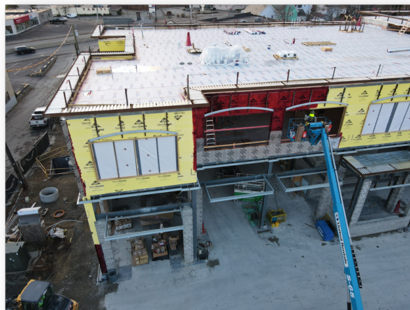
Photo of the active construction site taken using a drone on Friday, December 3, 2021 facing the north side of the building, along Bryant Street. Crews are priming the vertical air vapor barriers (shown in red) along the exterior walls of the building.
