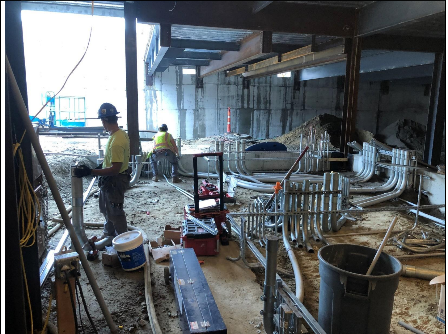
Electrical Room Underground Piping
