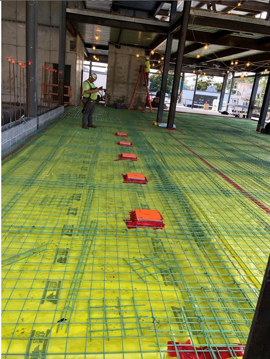
Electrical Floor Boxes
