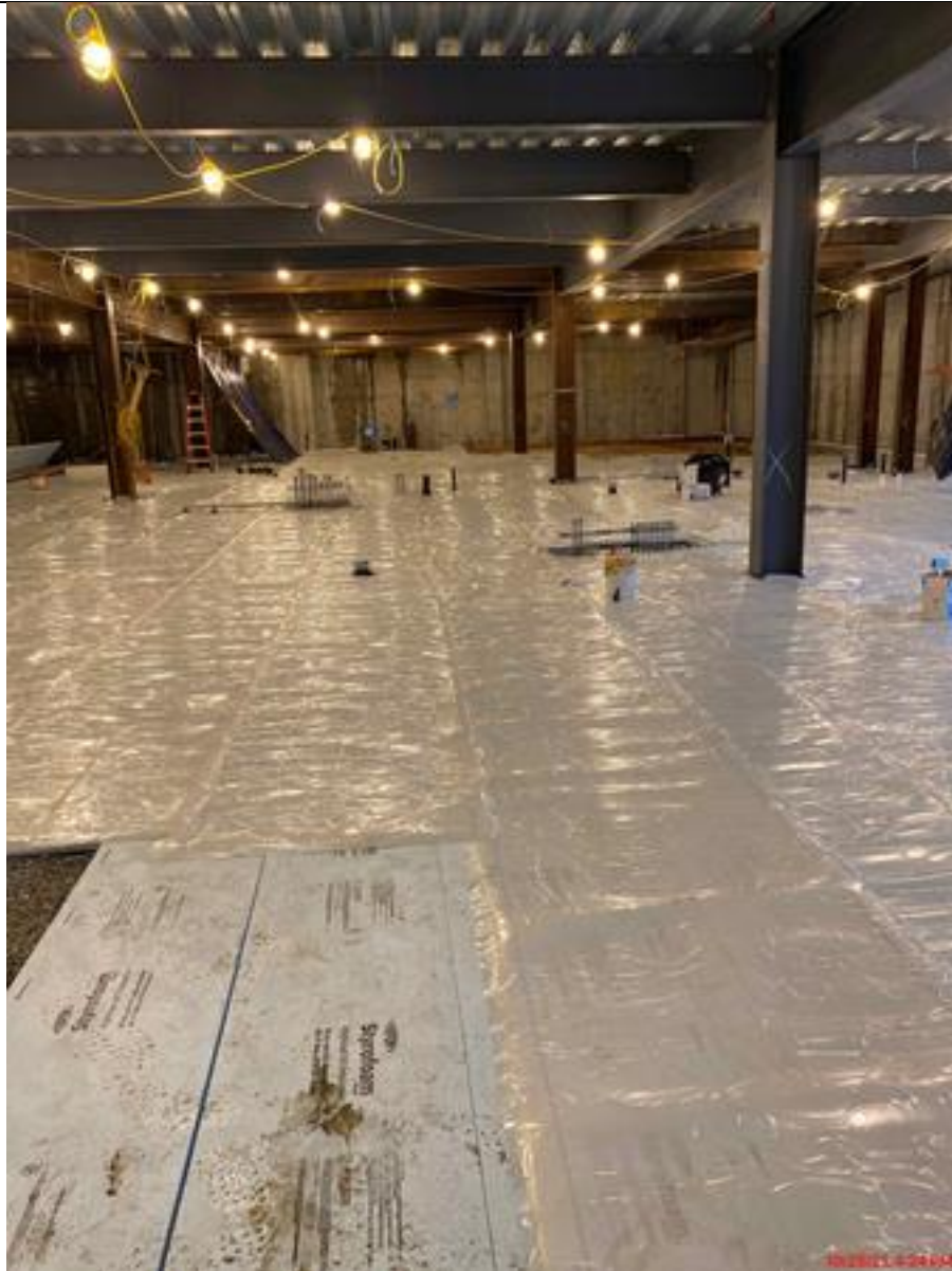
Basement Area Prepruf
