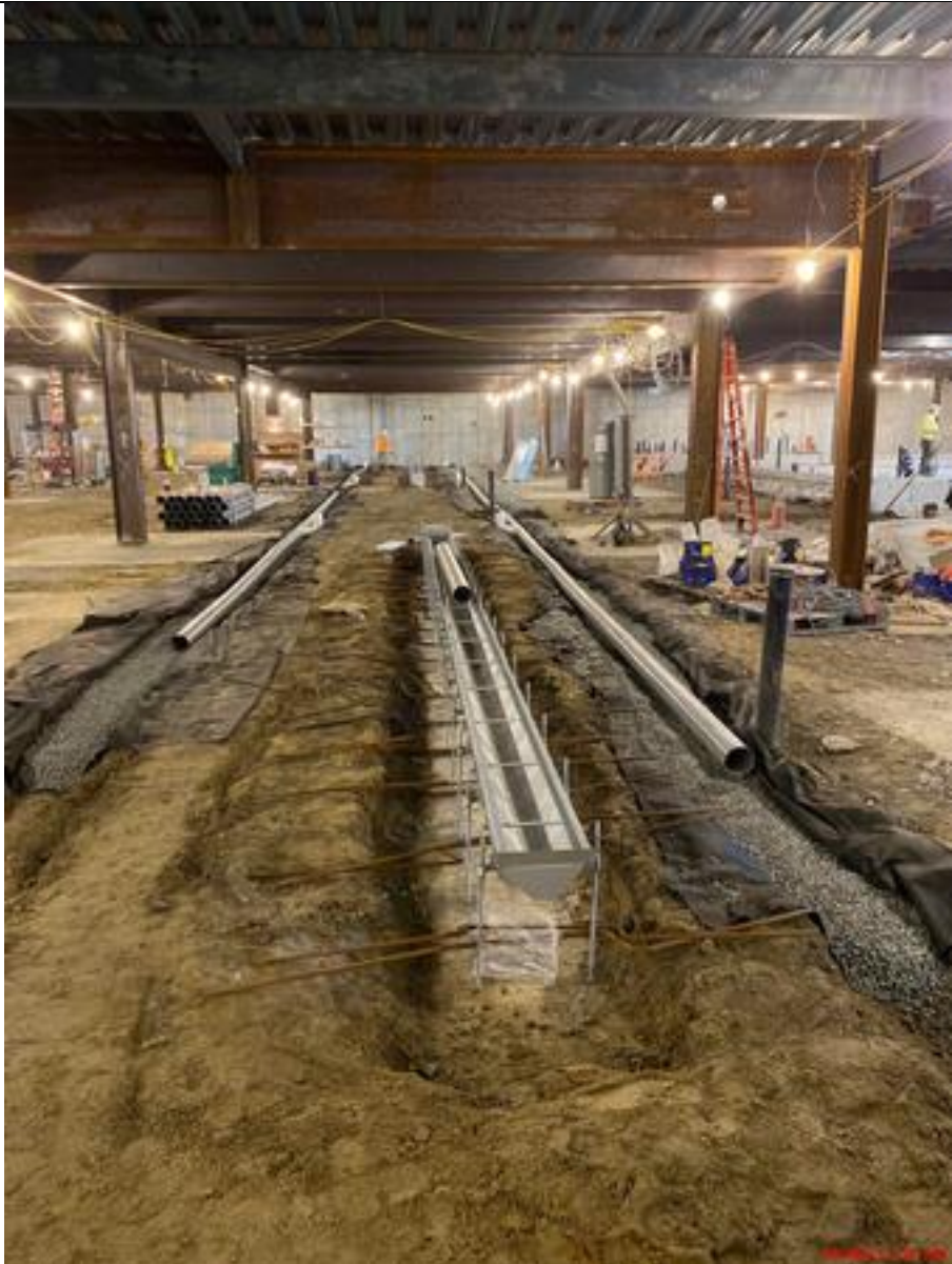
Garage Plumbing Trench Drains
