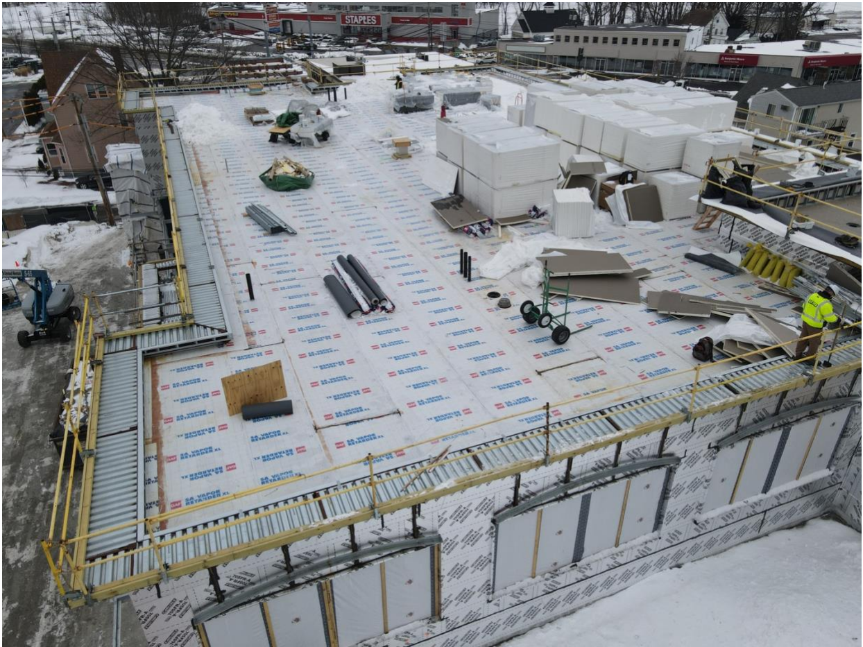
Caption: Photo of active construction site taken using drone on Tuesday, February 1, 2022. Roofing materials stored onsite (stacked white boxes to the right of the photo) will continue to be installed this week by roofing subcontractors.
