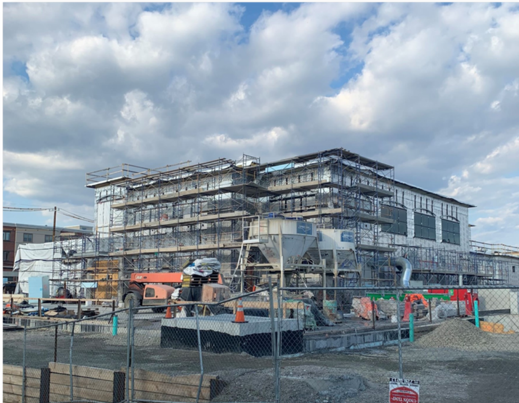
Caption: Photo of the active construction site, taken from the rear parking lot at Town Hall on Friday, March 18, 2022.
