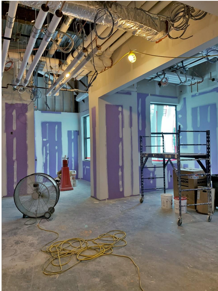
Caption: Photo of the drywall installation and painting underway within the second floor of the Police and Fire Stations as of Wednesday, May 18, 2022.
