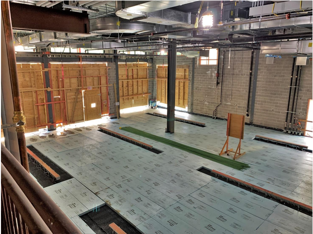
Caption: Photo overlooking the Fire Station maintenance bays taken from the mezzanine level as of Wednesday, May 18, 2022.
