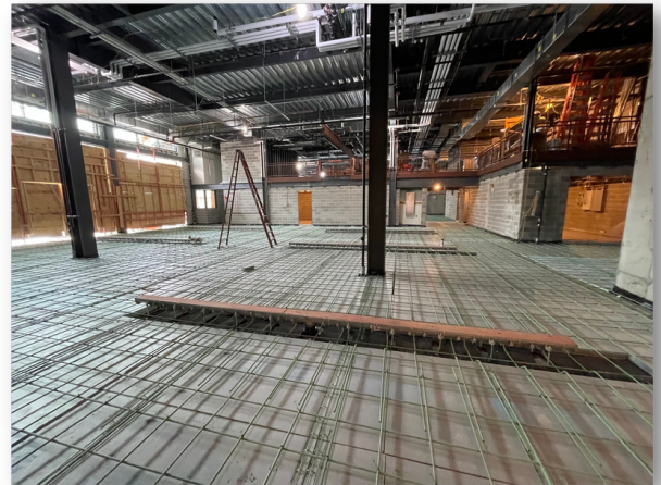
CAPTION: Photo taken on Wednesday, June 1, 2022, from within the Fire Department apparatus bays facing the mezzanine level. Contractors will continue to tie bottom reinforce each bay (rebar shown in the photo covering the entire floor of the garage) in advance of the placement of topping slabs.
