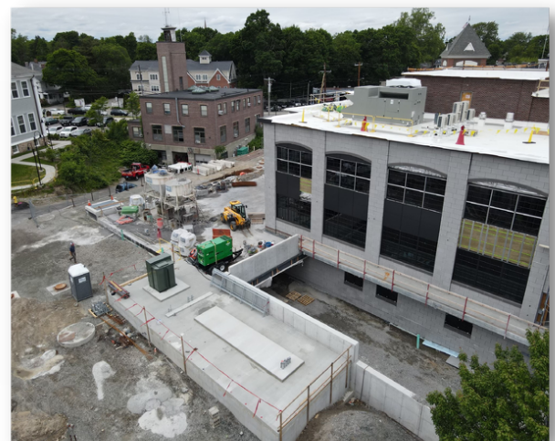
CAPTION: Photo taken on Wednesday, June 1, 2022 via drone overlooking the underground garage driveway entrance located along the south/southeast side of the building. To the left of the driveway entrance, at the bottom center of this photo, is the concrete pad for the generator that will be installed at a later date.
