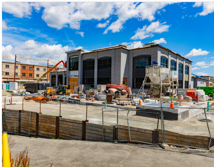
CAPTION: Photo of active construction site facing the south side of the building taken on Friday, June 10, 2022, from the north corner of the rear Town Hall parking lot.
