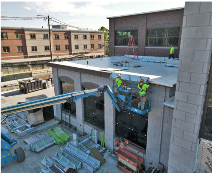
CAPTION: Photo of crews installing the parapet cap along the southern roof edge, taken by drone on June 23, 2022. Parapet caps help to create a uniform, finished look and prevent intrusion of water.
