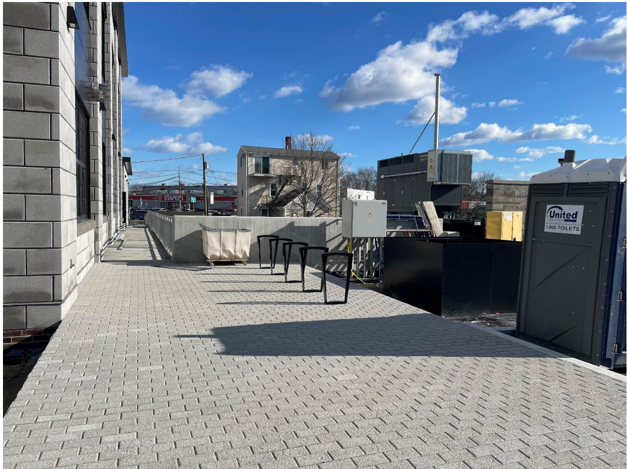
Caption: Stonework and bike racks installed outside new entrance to Public Safety Building along south side of building, taken on Thursday, December 1, 2022.
