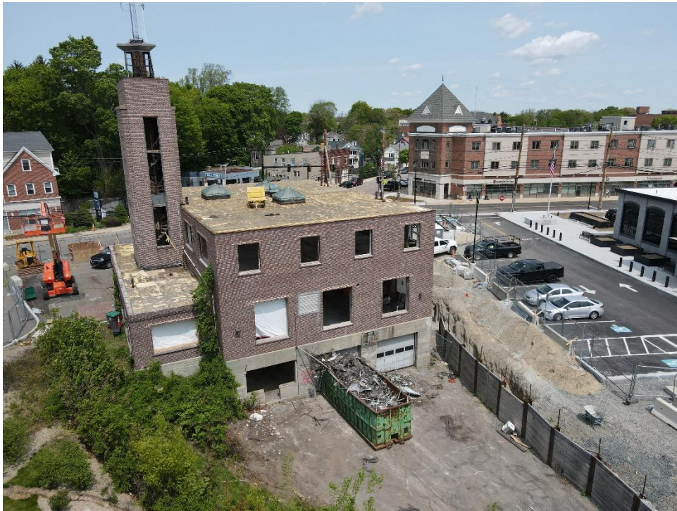
Caption: Photo of the rear of the former Fire Station taken on May 10, 2023 via drone during the abatement process. Crews started with the interior of the building and disposed of materials using the onsite dumpsters for disposal each day to a licensed offsite disposal facility.
