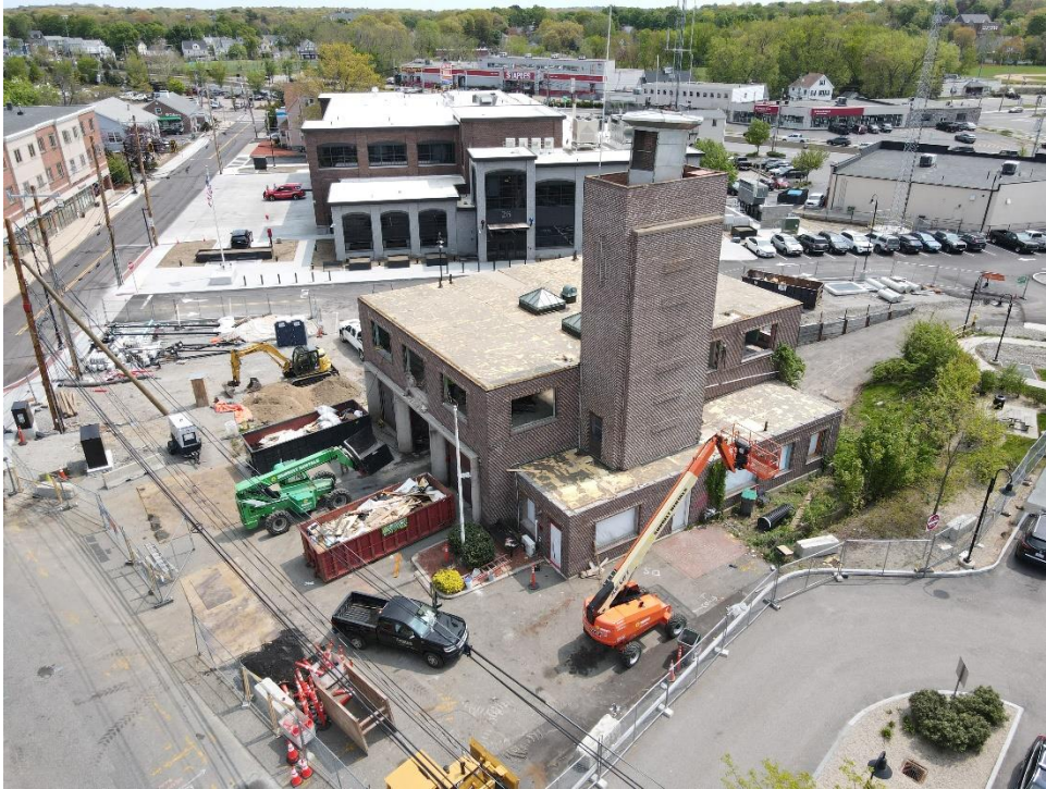
Caption: Photo of the apparatus bays to the former Fire Station taken on May 10, 2023 via drone during the abatement process. A crane is onsite to assist personnel with accessing upper levels of the building.
