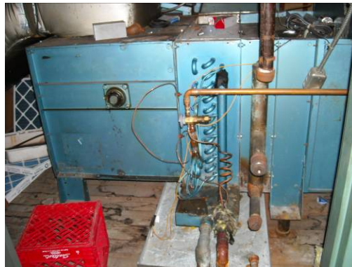
Attic – AHU (Serves Second Floor)
