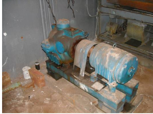
Compressor (Abandoned in Place)
