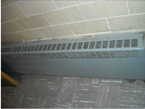
Steam Fin Tube Radiation Heating
