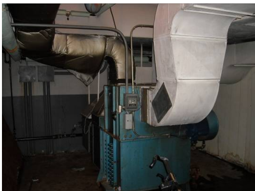
Basement – AHU (Serves First Floor)
