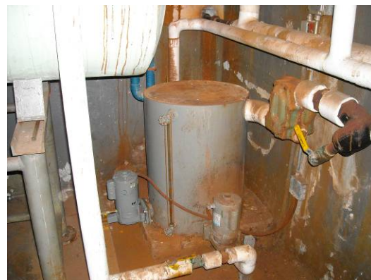
Boiler Feed Pump
