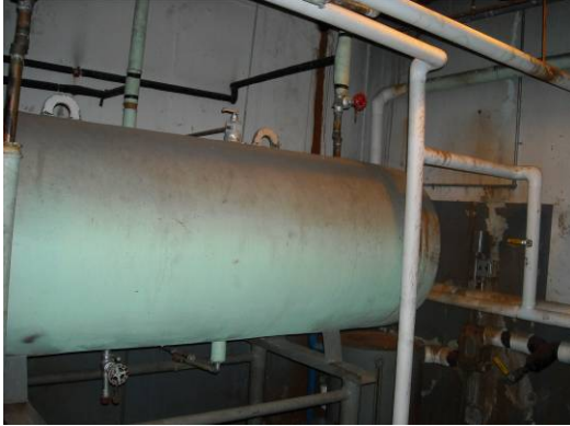
Illustration 1: Abandoned DHW Heater
