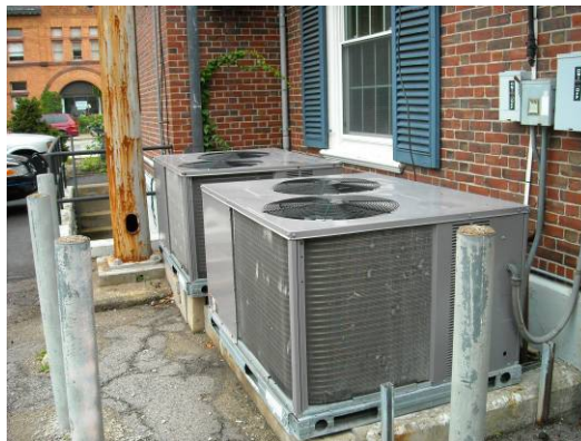
AHU Air Cooled Condensing Units
