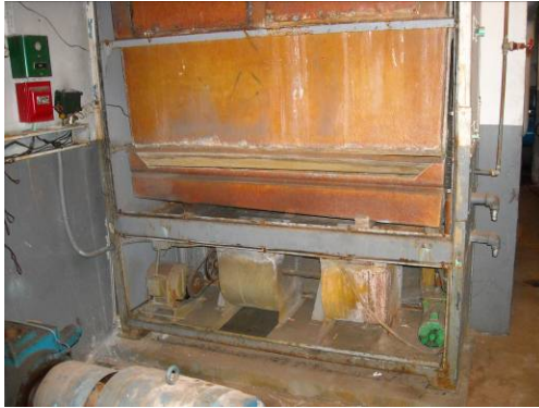
Gun Range AHU (Abandoned in Place)
