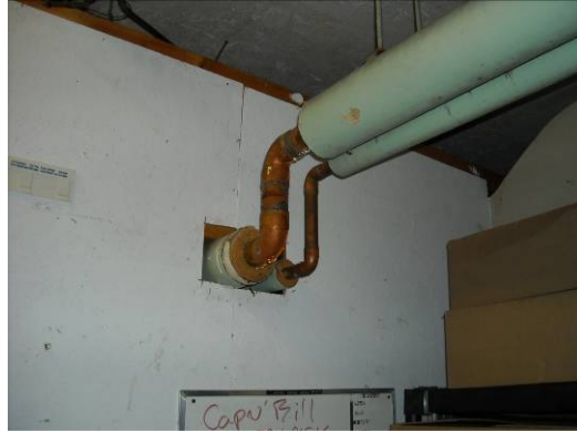
Steam and Condensate Piping Elbows without Insulation
