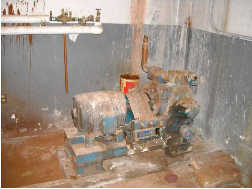
Compressor (Abandoned in Place)
