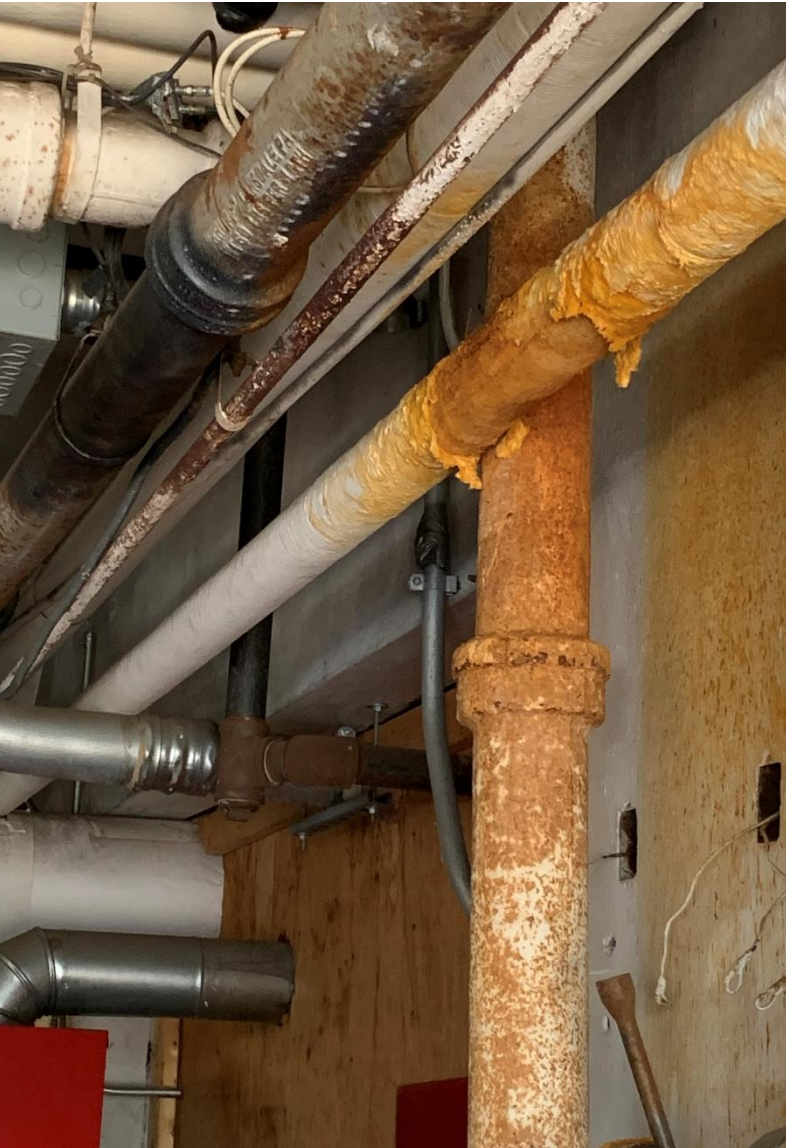
Deteriorated drainage pipes
