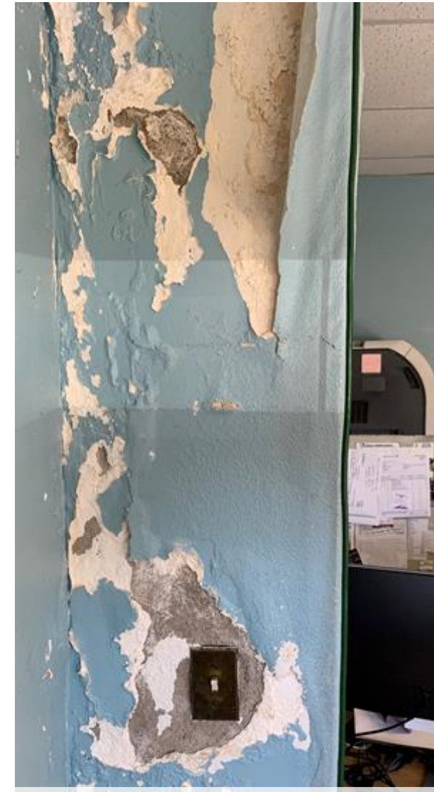
Perpetual water damage from tower
