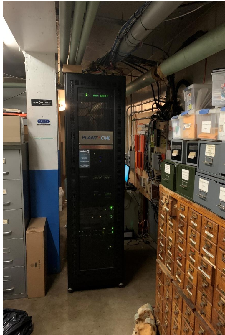
911 System Located in Storage Room with no HVAC
