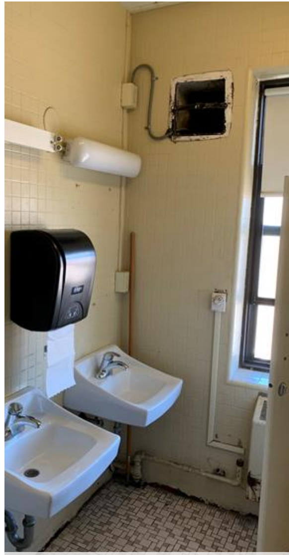
Restrooms are not code compliant and are not properly ventilated
