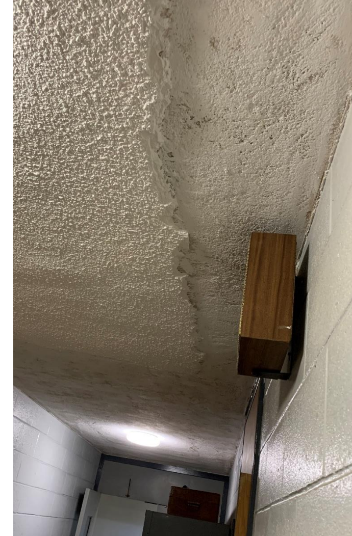
Deteriorating ceiling with material partially removed due to water damage and asbestos content.
