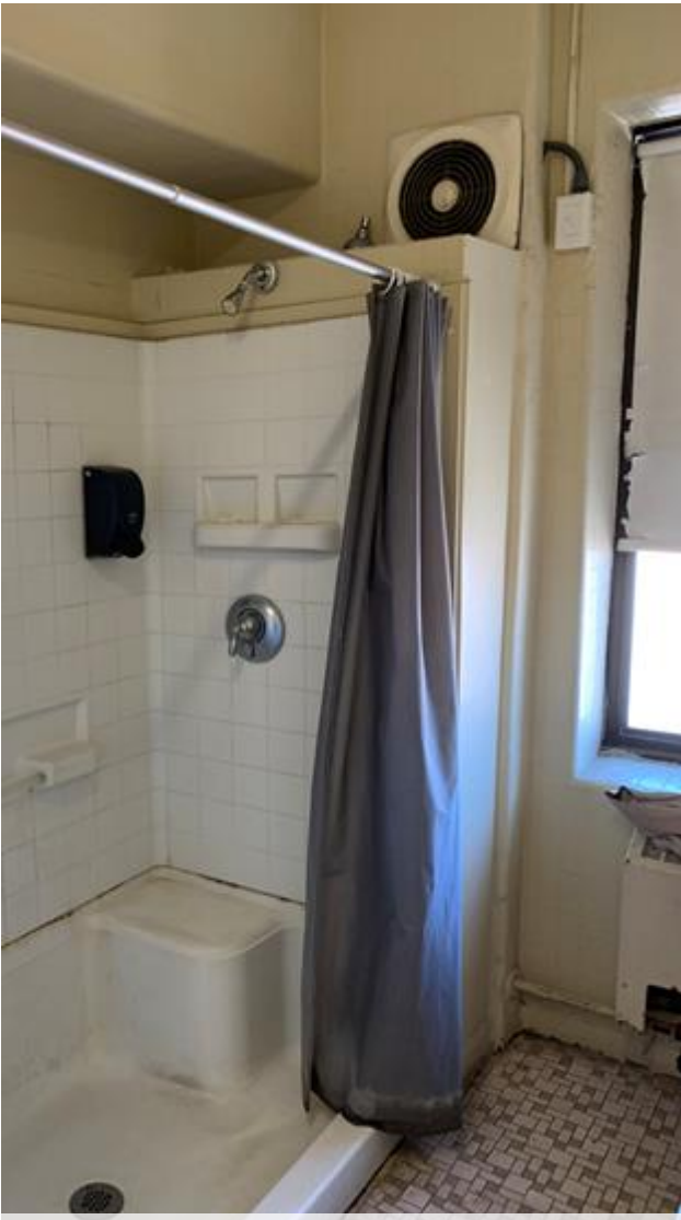
Insufficient number of showers to serve personnel
