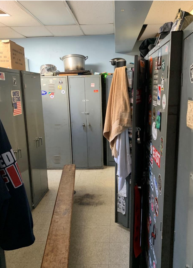
Locker room is undersized with inadequate storage space and no female locker rooms
