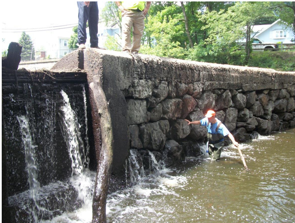
Photo 8: Seepage through face of dam and leakage through stop logs. Note scour measured downstream by approximately six foot long stick.
