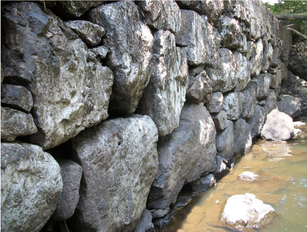
Photo 11: Large voids between stones making up downstream face of dam.
