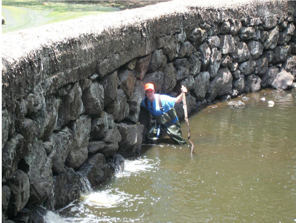
Photo 9: Large voids between stones on face of dam (no indication of soil movement).
