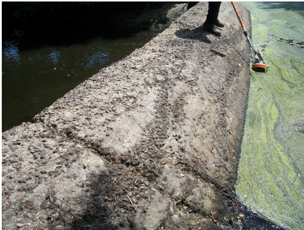
Photo 12: Scoured concrete along top of dam.
