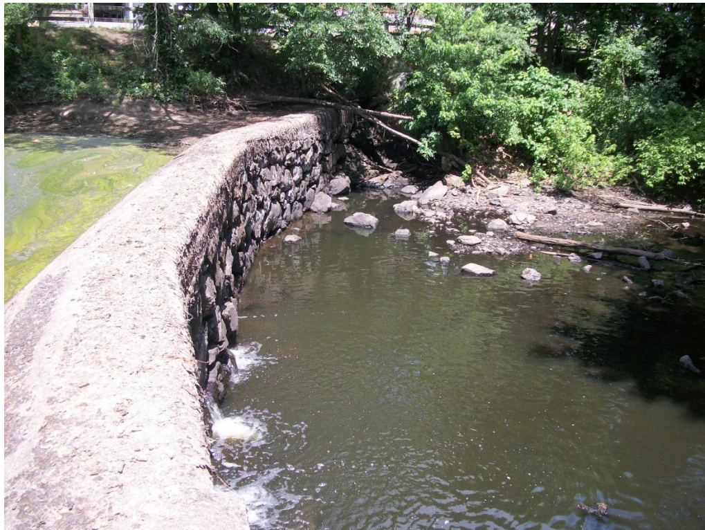
Photo 4: Woody vegetation at right abutment. Note seepage through face of dam.
