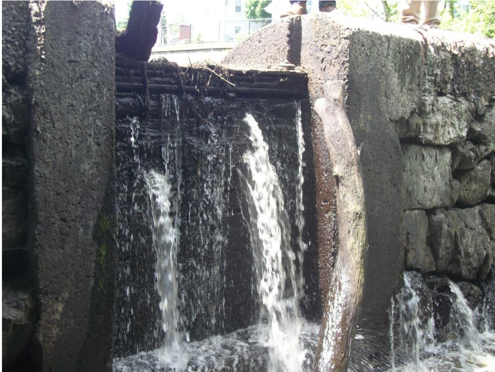
Photo 3: Leakage through the stop logs at the sluiceway.
