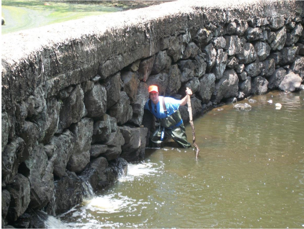
Photo 9: Large voids between stones on face of dam (no indication of soil movement).
